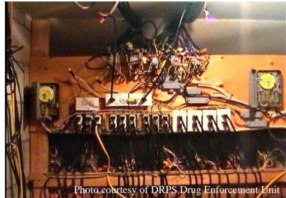
Police found an illegal hydro bypass in the Severn Street house.
